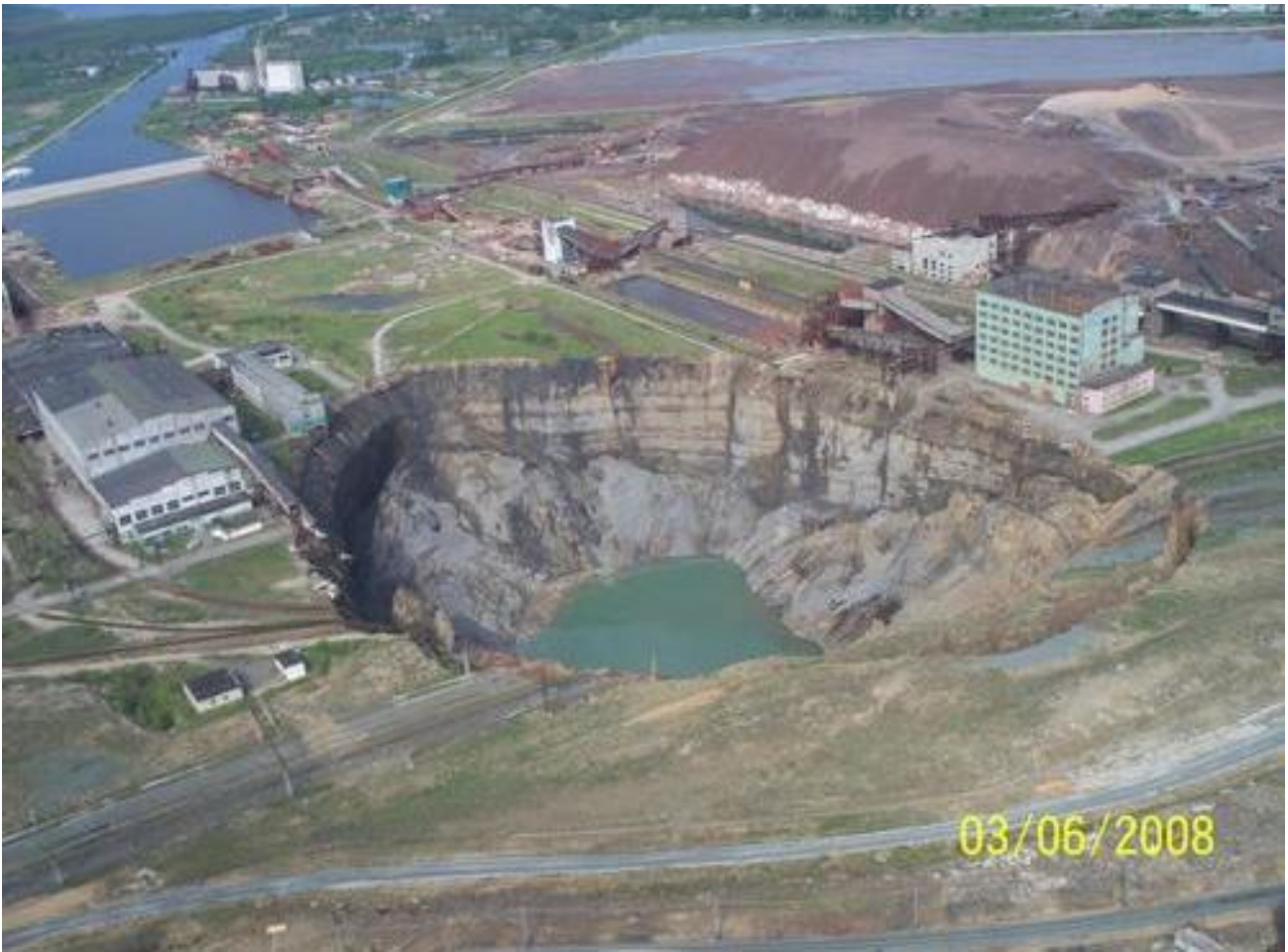
Figure 1: Sink hole at June 3 rd 2008 [Busch2008]
